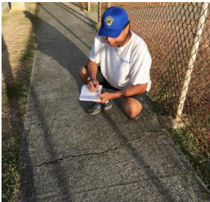
CIS Anthony Nakamura noting a cracked sidewalk.
